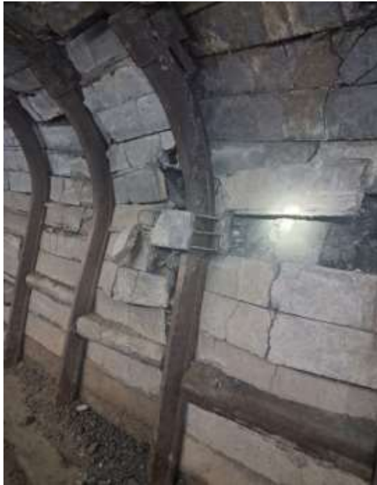
Figure 3. Local damage and cracking of lining elements caused by rock pressure.
