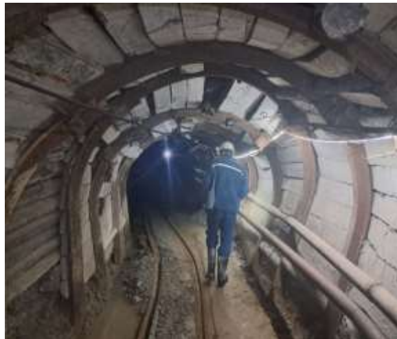
Figure 2. General view of an underground mine working supported by steel arch support.
